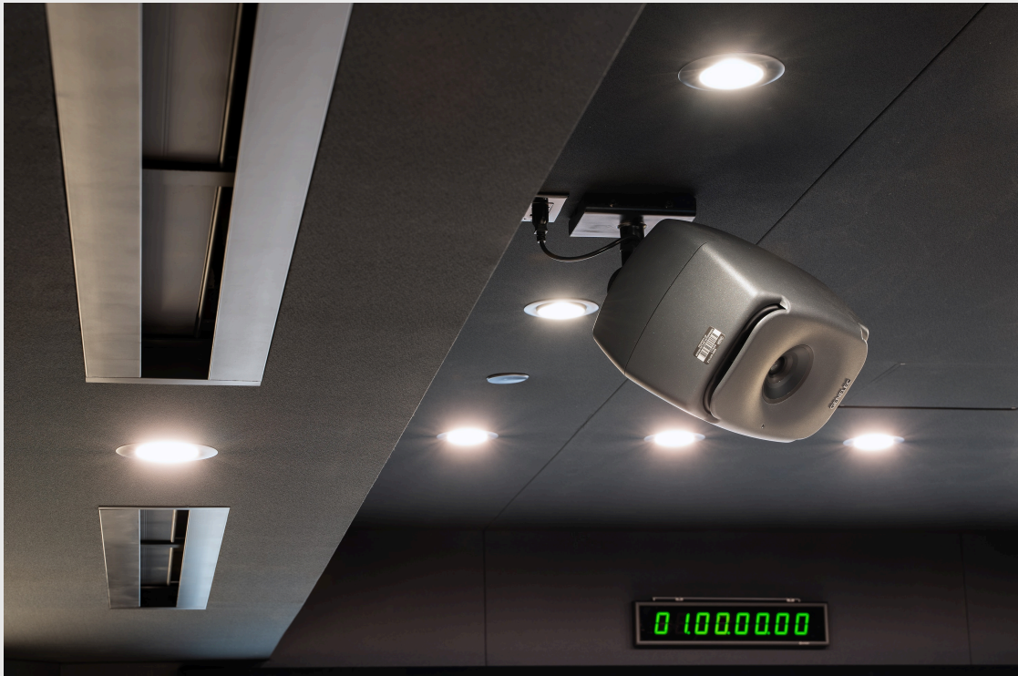
Overhead monitoring, soffits, lighting and ventilation were coordinated within the available height.
